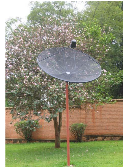
Satellite dish installed at National University of Rwanda Source: GEONETCast presentation (ITC, 2012)
